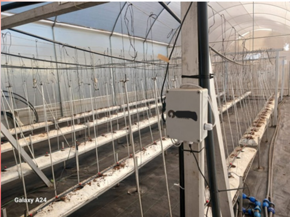
Smartgreenhouse planting structure for tomato production with sensor box controller
