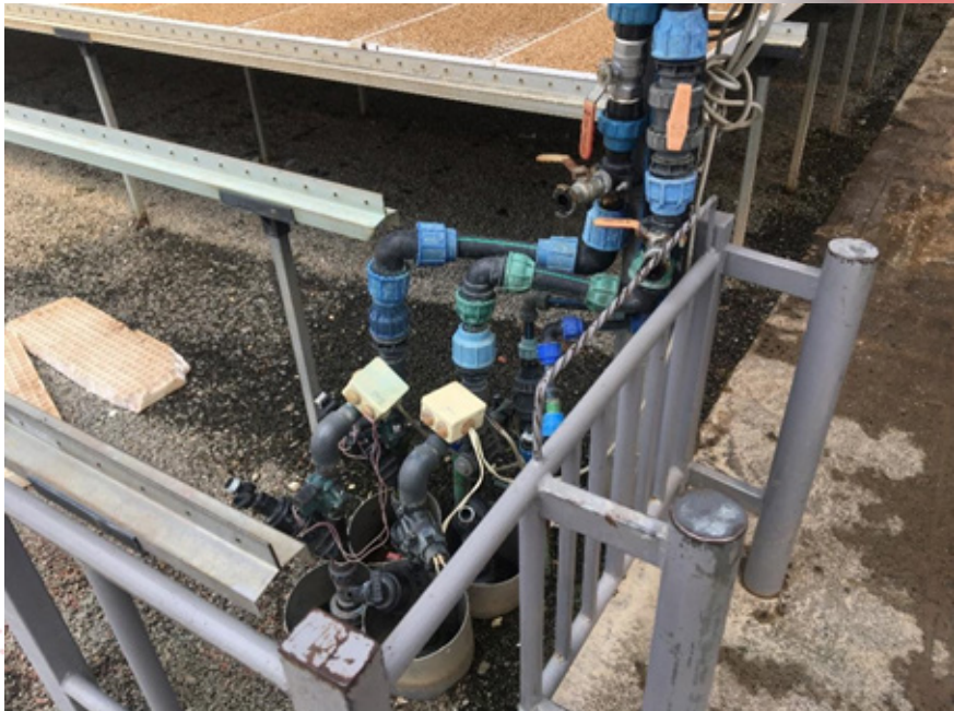
Fertigation chamber with sensor for irrigation and nutrient application
